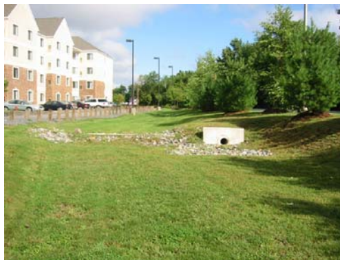
This infiltration basin collects and infiltrates runoff from the adjacent parking area.
